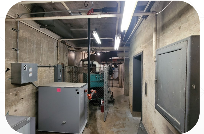
Fence Guard at Elevator
