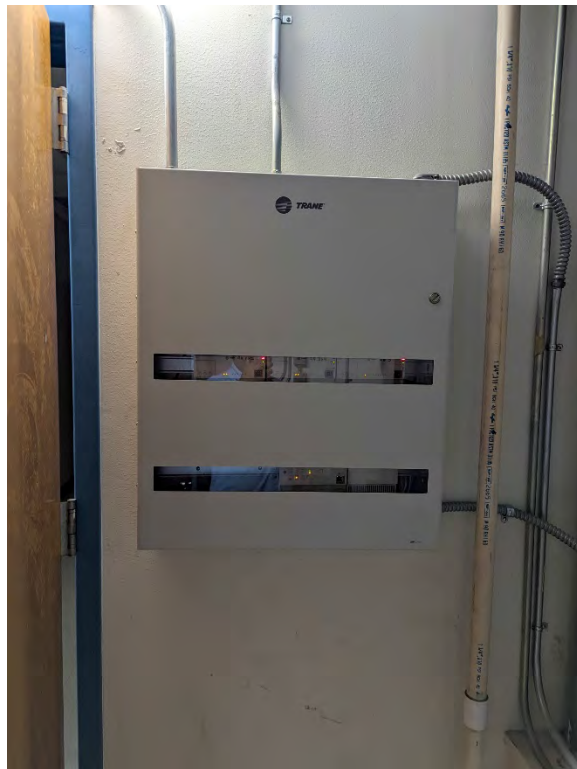
Figure 6. First floor controls cabinet
