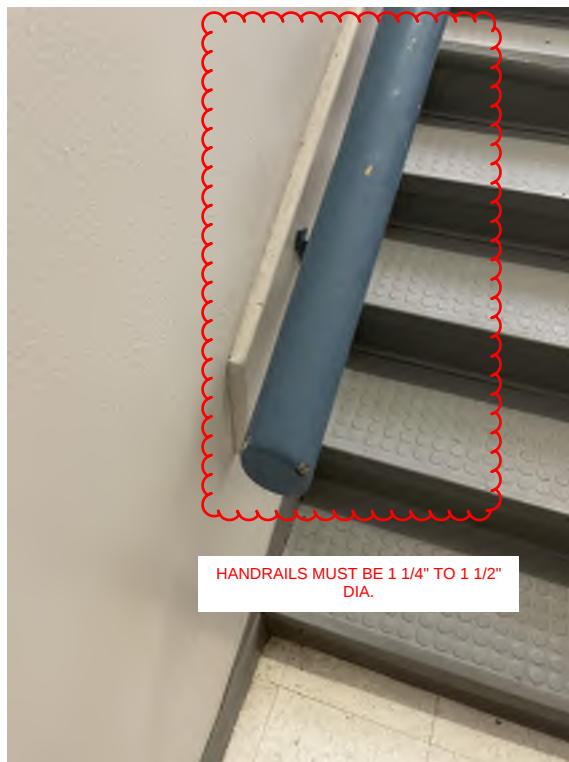
Figure 8: Stair handrails in First Floor Basement
