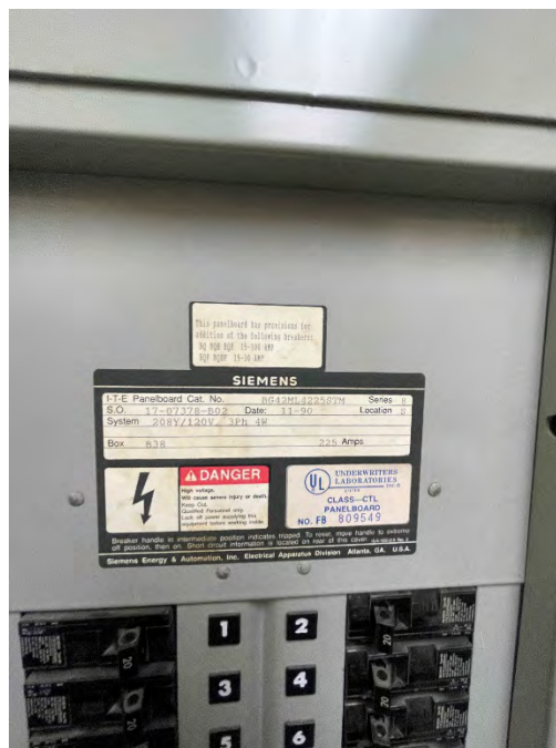
Figure 17. Panelboard nameplate showing a date of 1990
