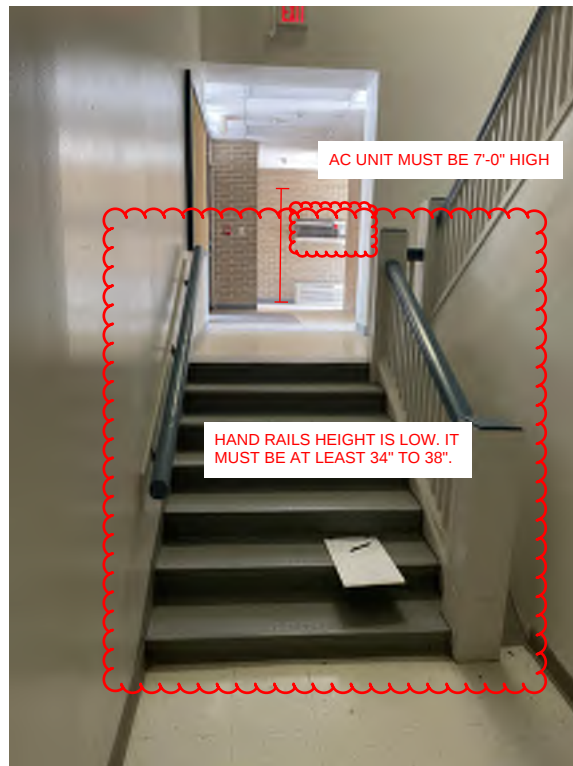
Figure 9: Stair handrails & AC unit not ADA complaint
