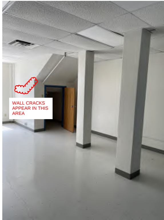
Figure 13: First Floor Basement Cracked Walls
